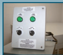
SPC switch box to control pump and fan operation
