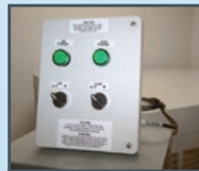
Switch box for control pump and fan operation
